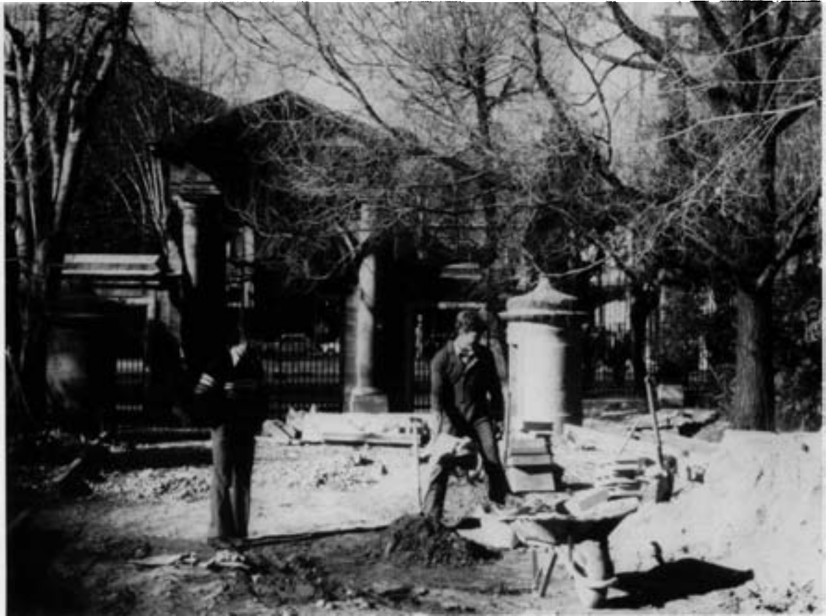
From 1974 until 1981, while it was being restored, the Madrid Botanic Garden had to be closed to the public. Plans developed by Leandro Silva Delgado, one of Spain's leading landscape architects, guided the restoration project. Shown here is construction work being done in February 1981 on the Ruiz and Pavón Pavilion, just inside the Puerta del Rey, or Royal Gate. (The Gate and the Paseo del Prado are in the background.) Photograph courtesy of J. Walter Brain.
