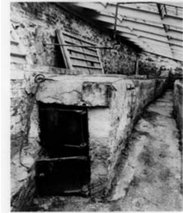
The earliest greenhouse at "The Vale," Theodore Lyman's estate in Waltham, Massachusetts, probably dating from 1804. This photograph shows the firebox and the horizontal flue for heating. Kirk Boott's greenhouse probably was quite similar. Courtesy of The Society for the Preservation of New England Antiquities.
