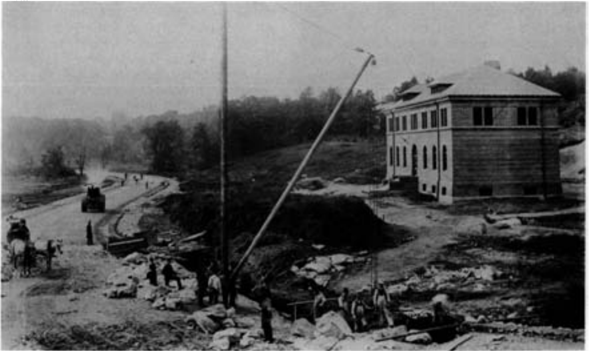
The Hunnewell Building under construction in 1892. All photos are from the Archives of the Arnold Arboretum.
